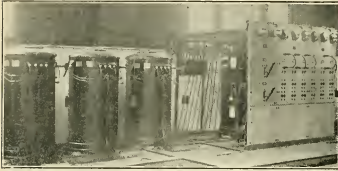
SWITCHBOARD (A), CONTROLLING ALL OUTSIDE CIRCUITS, AND THE SERIES TRANSFORMERS FOR THE ARC-LIGHT CIRCUITS.
